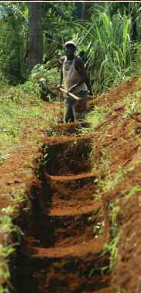
Rwanda, Gatanga, February 2007 Food for work project, terracing for erosion control project in Gatanga, Bugesera district.
