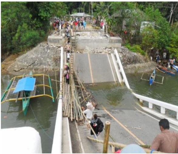
A collapsed bridge in Bohol.
